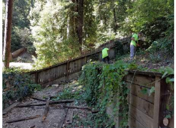
Slopes greater than 50% required careful hand digging during the Geoflow drip system installation
